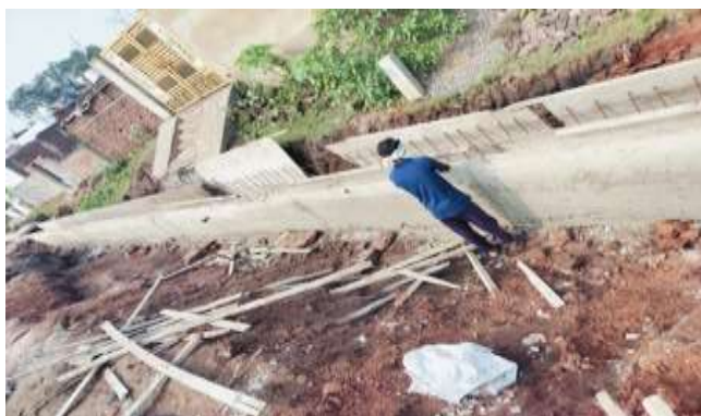
Drain at Siltara
